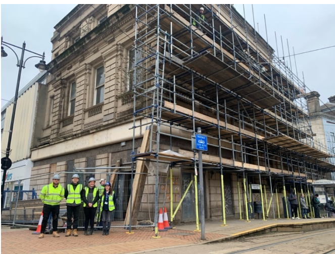
Left to right: Arron Rose , Site Manager, Andy Hare , Construction Manager, and Amy Stamford , Commercial Manager from Pinnacle Conservation and Rebecca Sleight , Senior Building Surveyor from Rider Levett Bucknall
